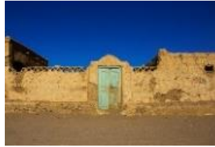
FIGURE 20. Cob wall plaster (zibala) easily washed away by rainwater
